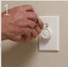
Turn off breaker
